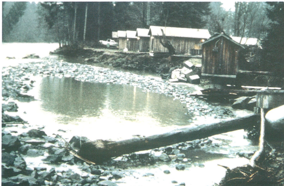
Channel bank erosion has lead to lost ground
