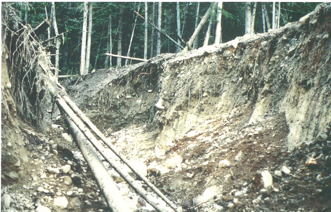
An example of severe channel erosion
