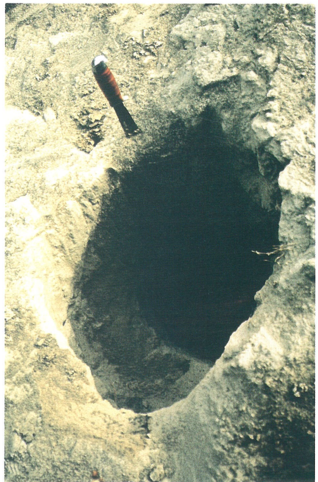
Exit hole of underground water (piping)
