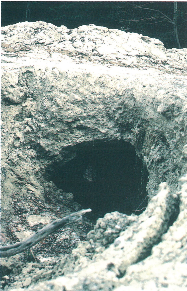
Exit hole of an underground water pipe
