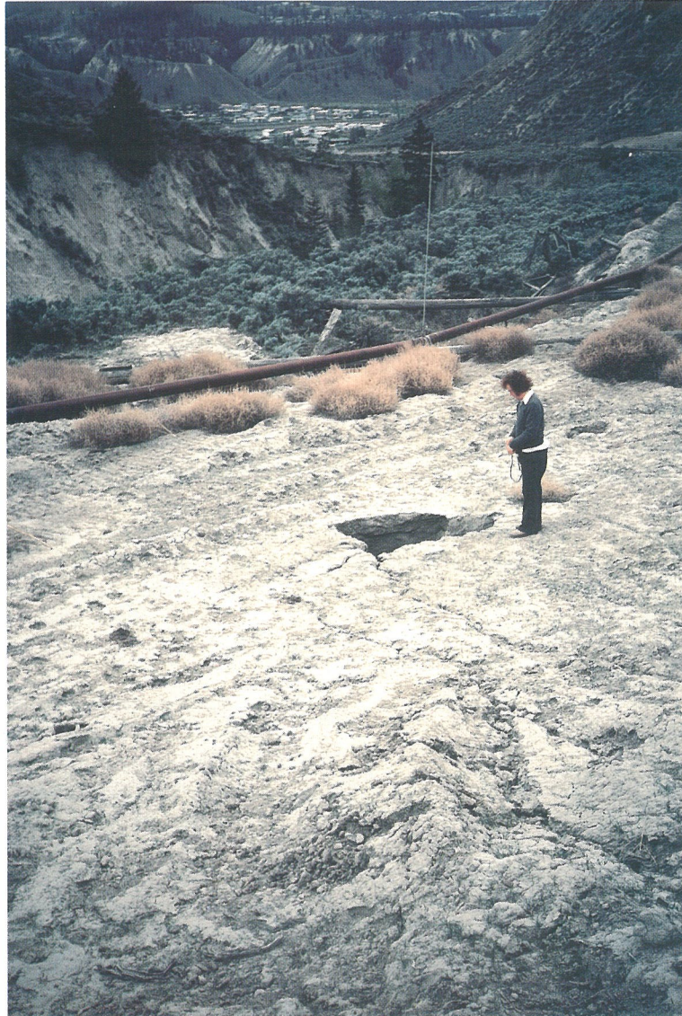
Sink hole due to leaking water pipe
