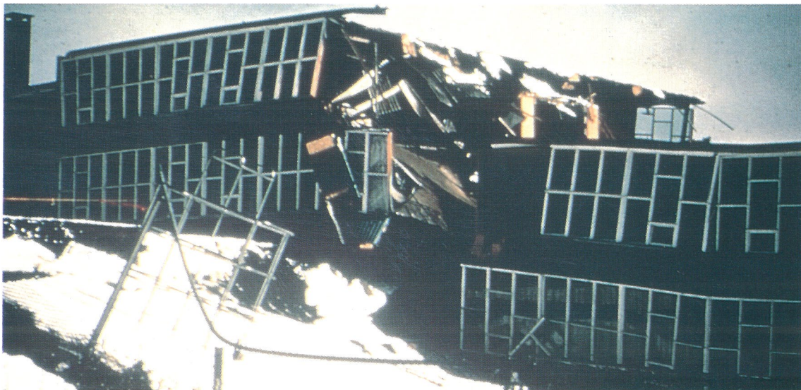
A school in Alaska heavily damaged in the 1964 Alaska earthquake
